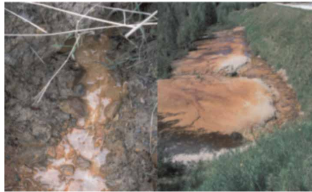
Figure 3 | Examples of seepage water sampling points at showing the upper seepage area at the toe of the upper section of the dam (Heikkinen 2009).
